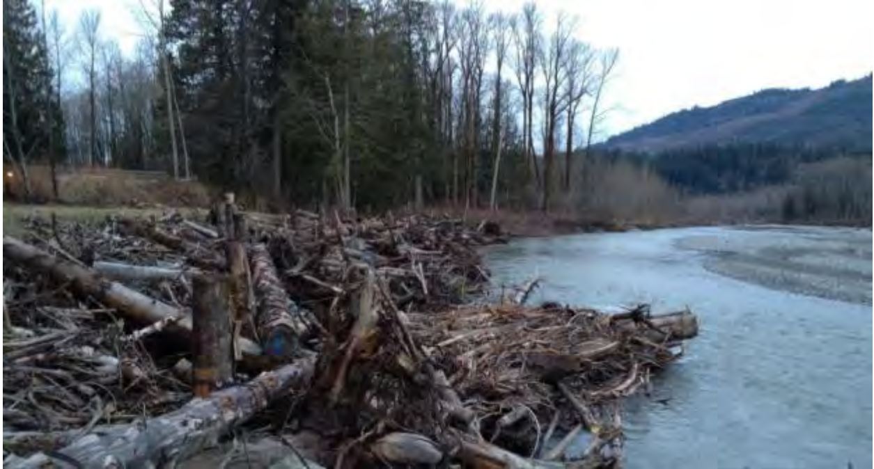
Figure 17. An engineered, complex wood revetment built by the Lummi Nation along the South Fork Nooksack River. The structure is stabilized with timber piles and rock collars creating a rough streambank very different than traditional rock revetments such as riprap.
