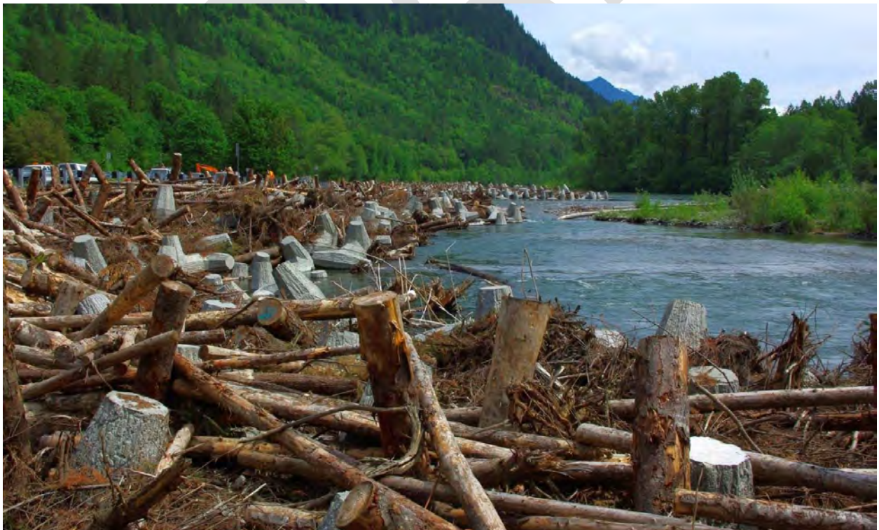
Figure 18. An engineered, complex wood revetment constructed by WSDOT on the Skagit River to protect SR 20 at milepost 100.7. This structure is stabilized with concrete dolo anchors and ballast due to site constraints. Photo from WSDOT (2014).
